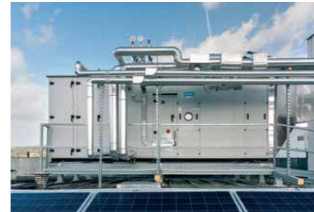
Figure 25: Example of an outdoor installation
